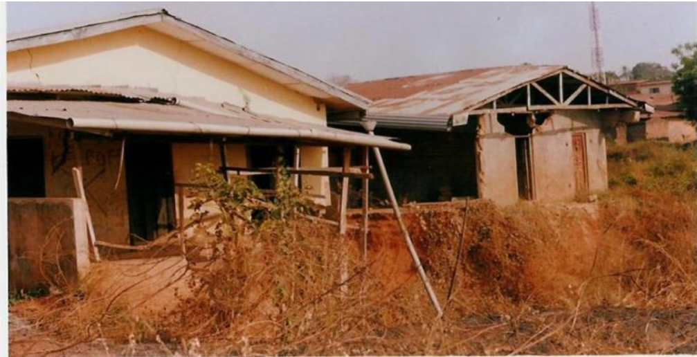
Plate 1: Erosion threat to residential land use at Iyekhei quarters
