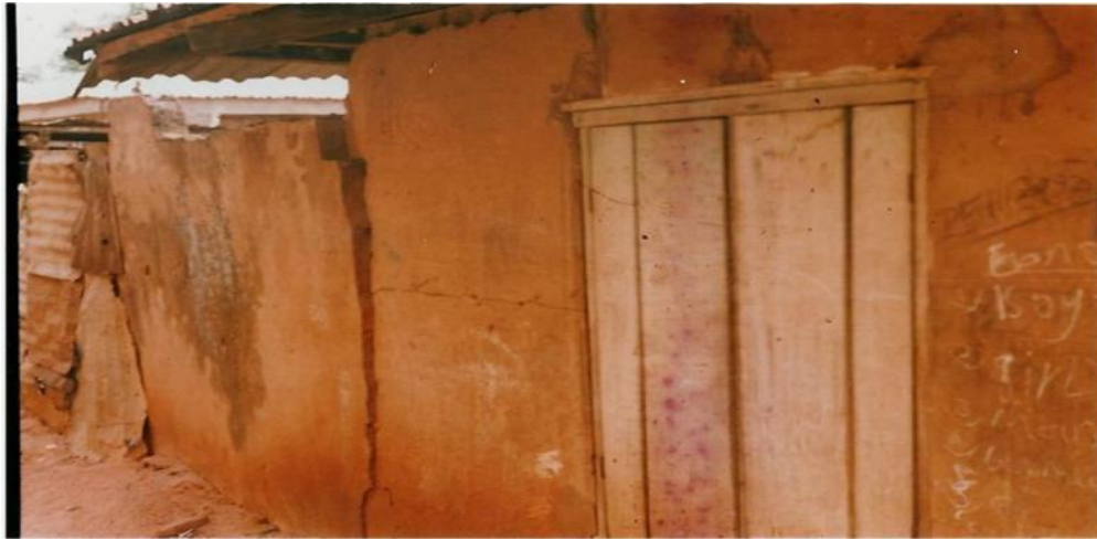
Plate 4: Cracks on Residential Land use at Igbei Quarters
